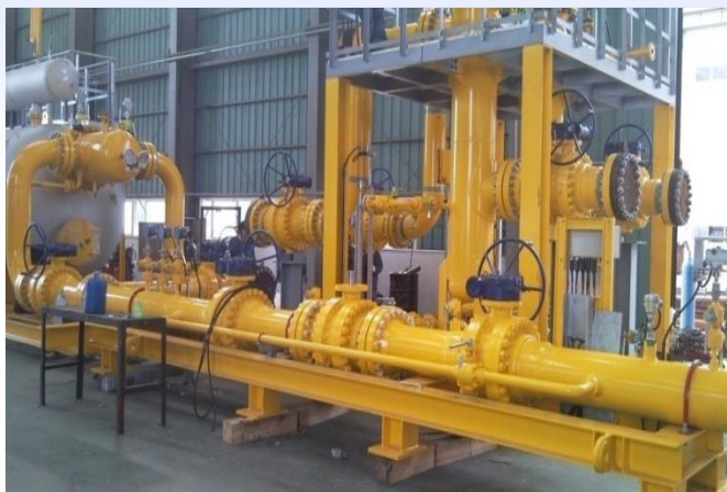
SAMRA POWER STATION PHASE-III, SIMPLE CYCLE PROJECT
